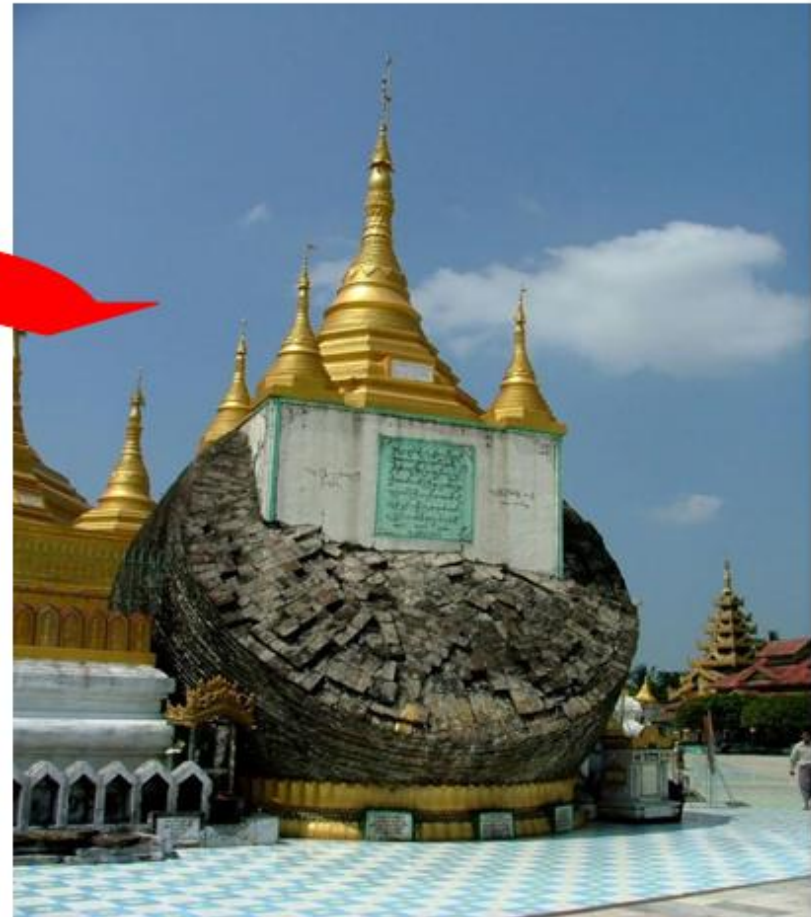
Top portion of the pagoda fallen down by 1917 Bago Earthquake
