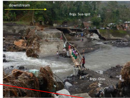
Fig. 11. Damaged culvert bridge connecting Brgy. Sua-Igot and Brgy. Oras
