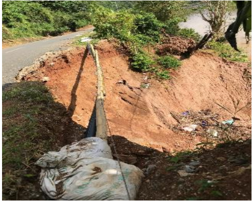
Damage on mainline distribution network of Nam Papa in Ngoy district of Luang Prabang province
