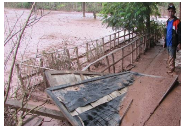
Damaged school building and equipment at Sanamxay, Attapeu. Photo credit: Save the Children International staff
