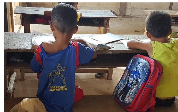
Superheros of Laos – Children are staying in a partially damaged building with hazardous structural damages in Savanakhet. Photo credit: Tara I.M., Plan International Australia.
