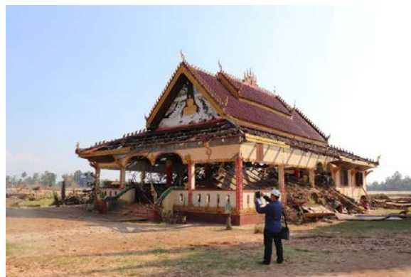
The damage at Vat Ban Hinlad (1), Sanamxay District, Attapeu Province. Photo credit: Souvanhnikone Phatanh
