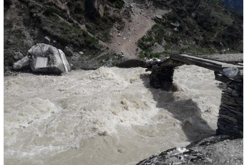
Figure 12. Bridge damaged by the Flood
